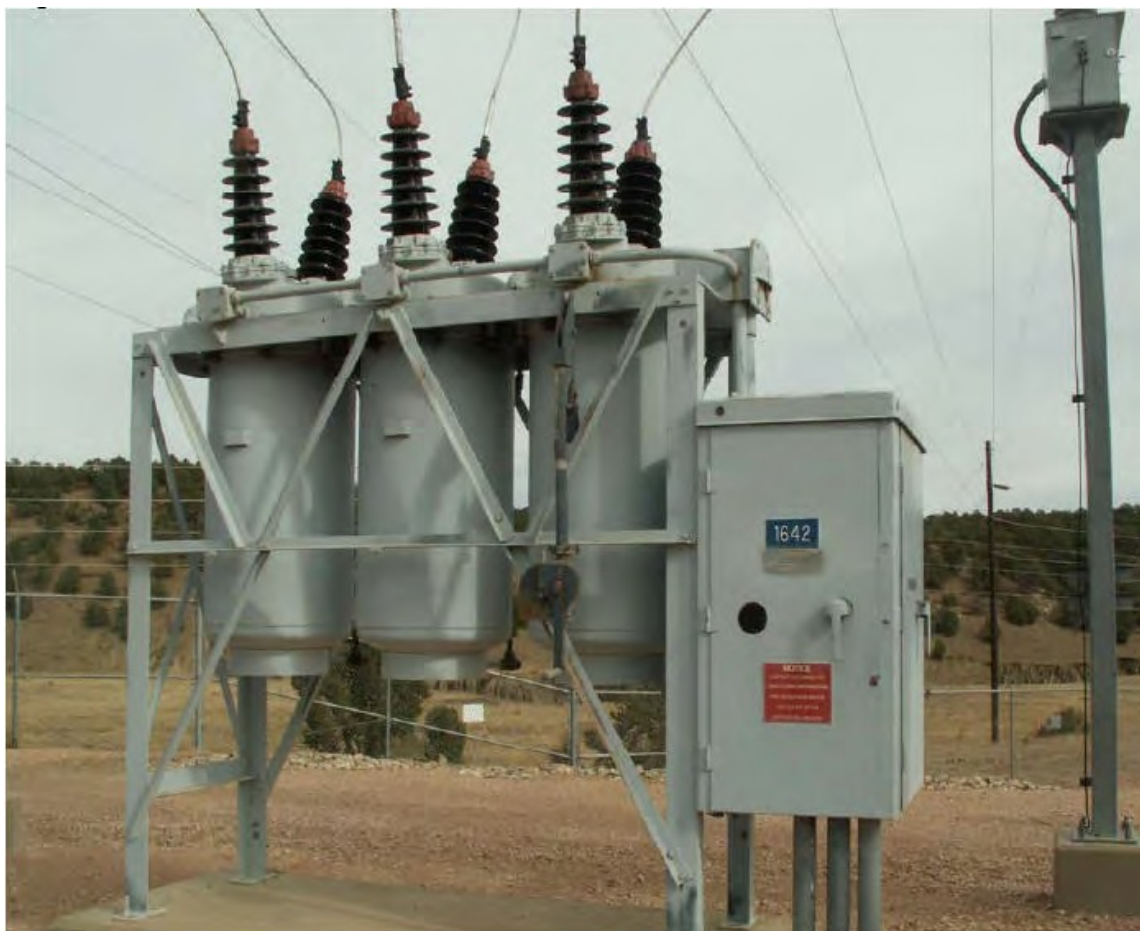
Figure 5.2: 46kV Oil Circuit Breaker
