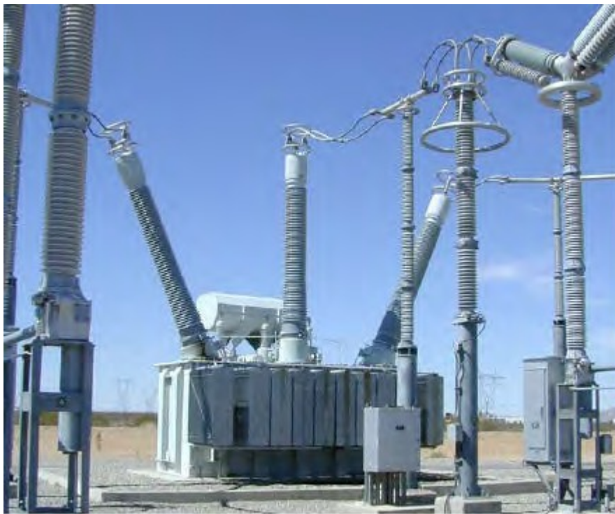
Figure 5.10: High-Voltage Line Reactor (500kV)
