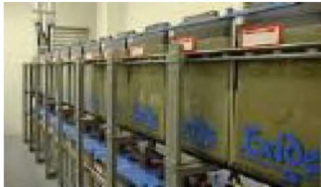
Figure 5.18: Substation Battery Bank
