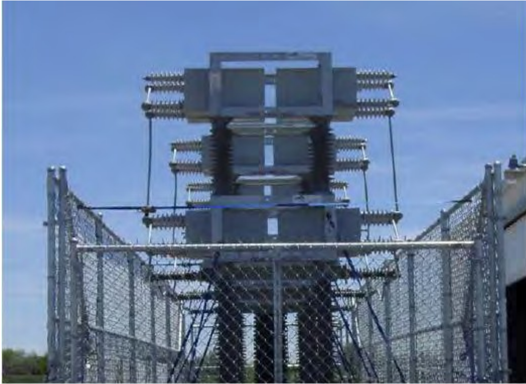
Figure 5.9: High-Voltage Capacitor Bank
