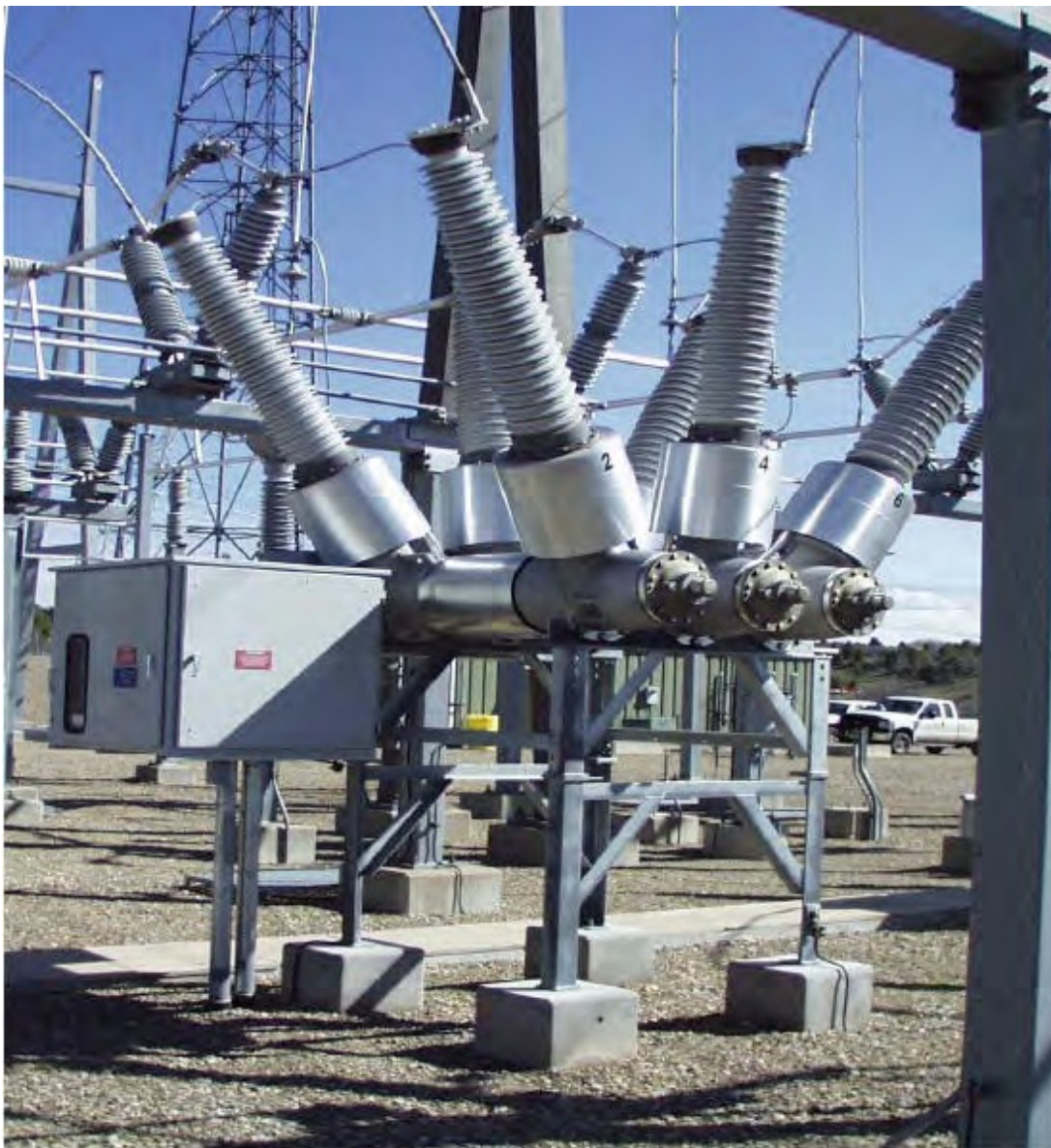
Figure 5.6: 115kV Gas Puffer Circuit Breaker
