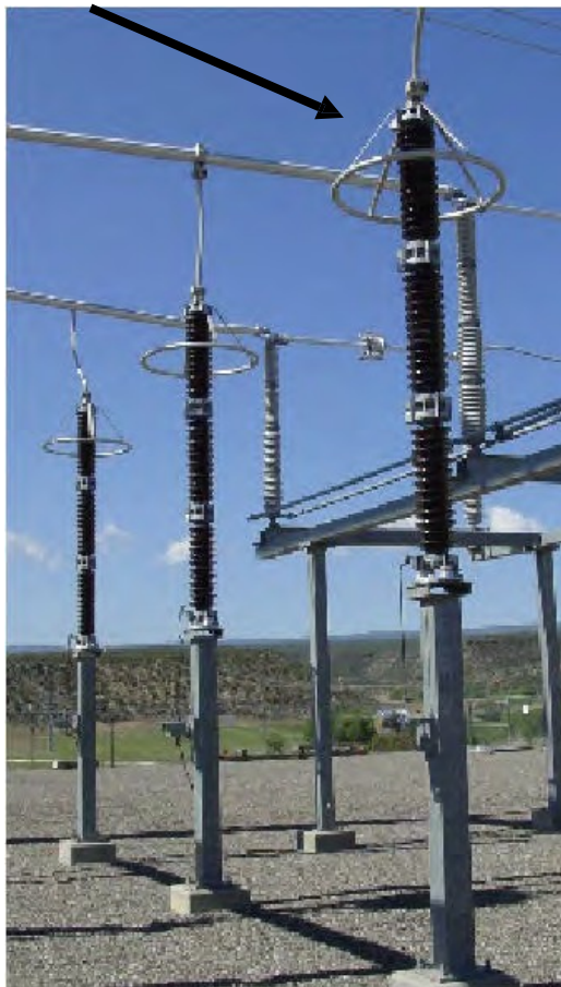
Figure 5.15: High-Voltage Lightning Arrester on High-Voltage Bus
