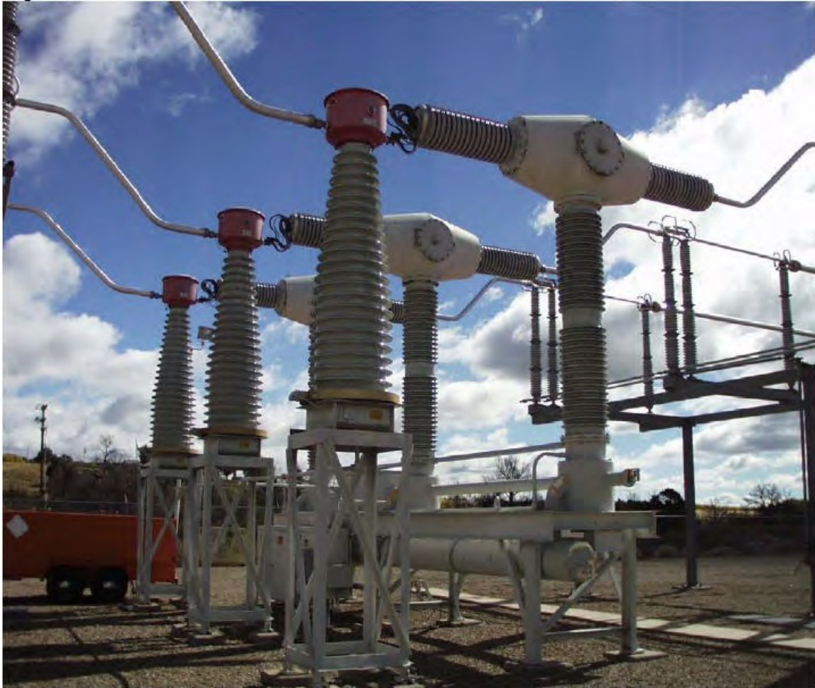
Figure 5.5: 230kV Gas Blast Circuit Breaker
