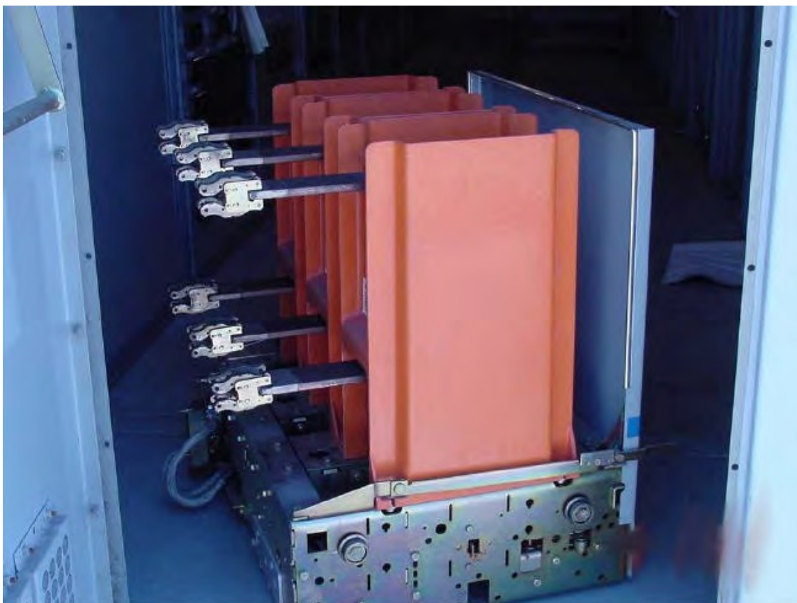
Figure 5.7: 34.5kV Vacuum Circuit Breaker
