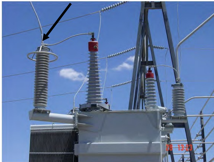
Figure 5.14: High-Voltage Lightning Arrester
