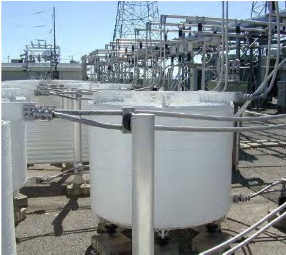
Figure 5.11: Low-Voltage Tertiary Reactor (13.8kV)
